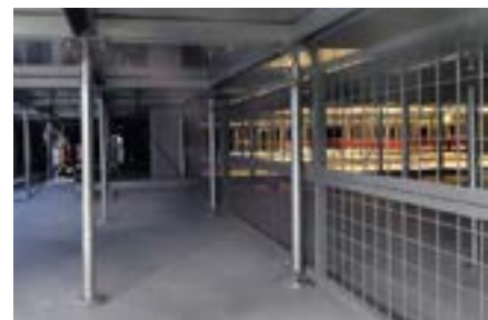
An example of mesh infill between the building floor and the computer floor.
